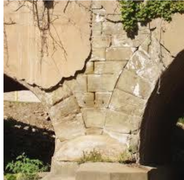
Example Bridge Deterioration
